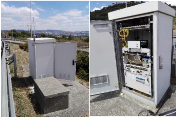
Figure 6 – Example of a Brisa’s roadside equipment
