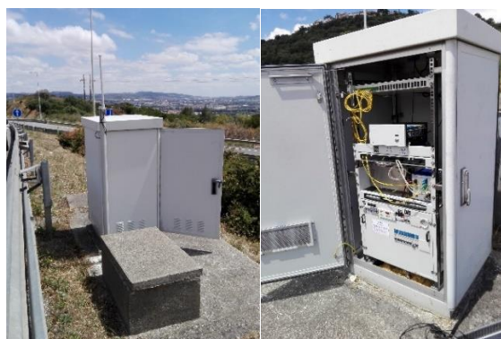
Figure 6 – Example of a Brisa's roadside equipment
